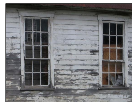
Photo 9: Damaged Exterior Envelope
