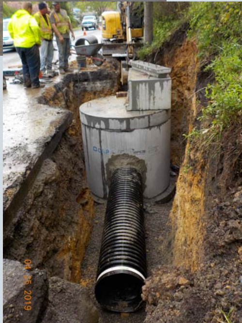
US 220 McMullen Hwy Southbound Lane New I_3-2 Inlet Modified SHA COG Inlet Approx. 8 Foot Depth
