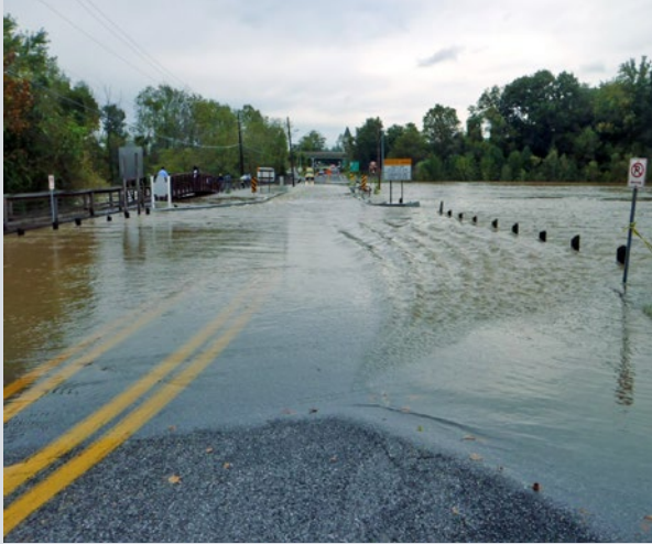
Water Street Bridge (MD 717) in Prince George's County floods multiple times per year.
